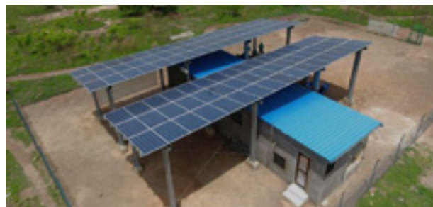
Figure 2: Installation de micro-réseau de 54 kW à Kudorkope, Ghana Source: Volta River Authority, Ghana.
